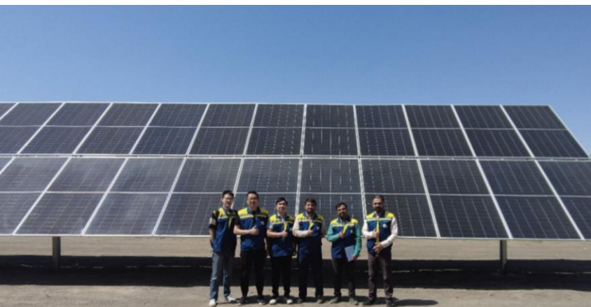
Arab Emirates, 20MW, Tracking Mounting System
