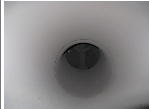
Inspection area No. 7: take photo of exh. valves from the exh. gas receiver side. Comment:
