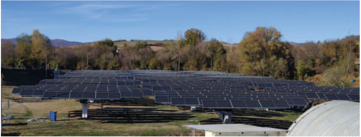
640kW Commercial & Industrial project
