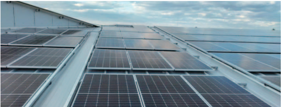
120kW Industrial Project
