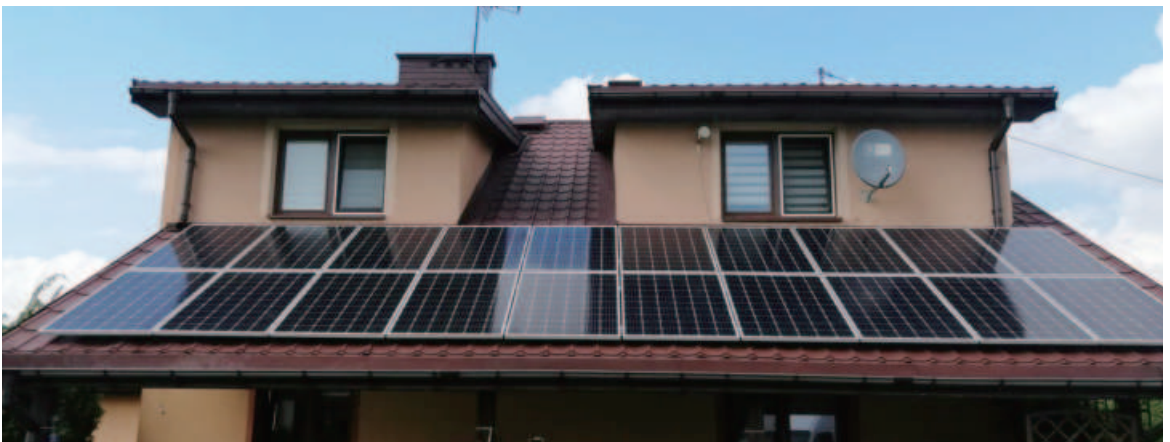
8kW Home Photovoltaic Project
