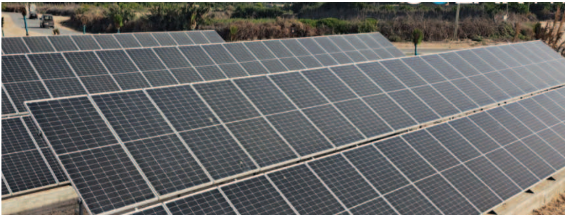
295kW PV Power Station Project
