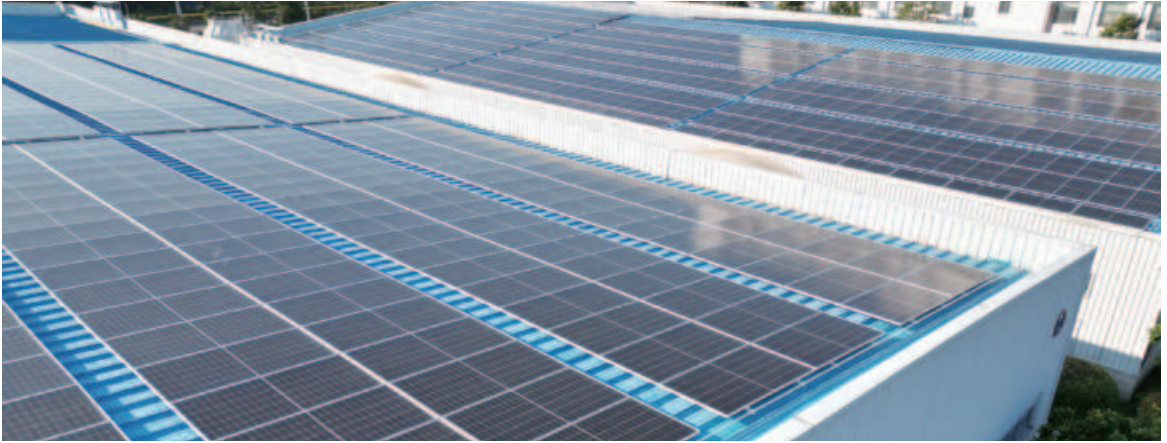
1MW Industrial Roof Project
