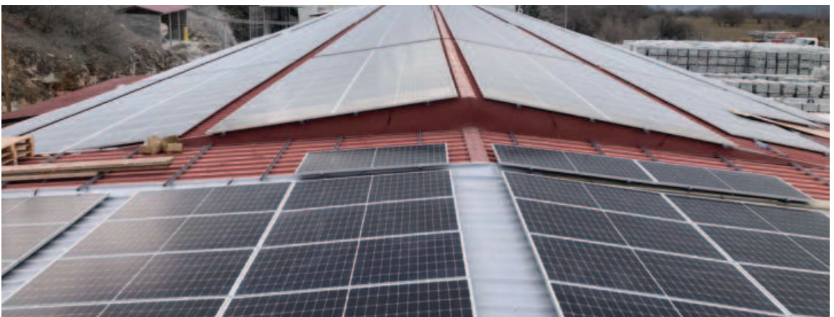
700kW Industrial Roof Project
