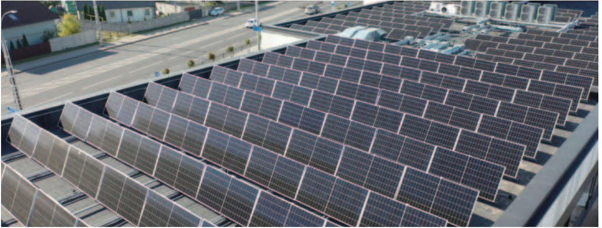
100kW Industrial Roof Project
