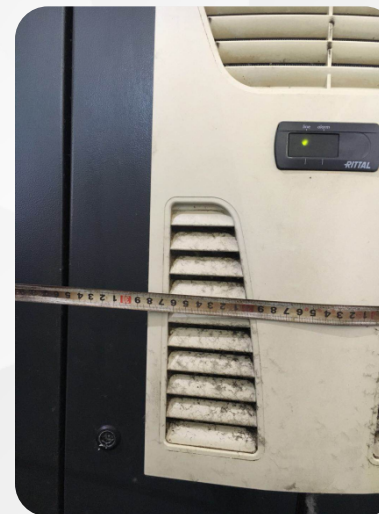
3-The width of the AC to be replaced.
